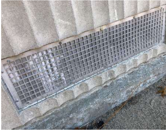
Unit Ventilator Outside Air Intake Obstructed
