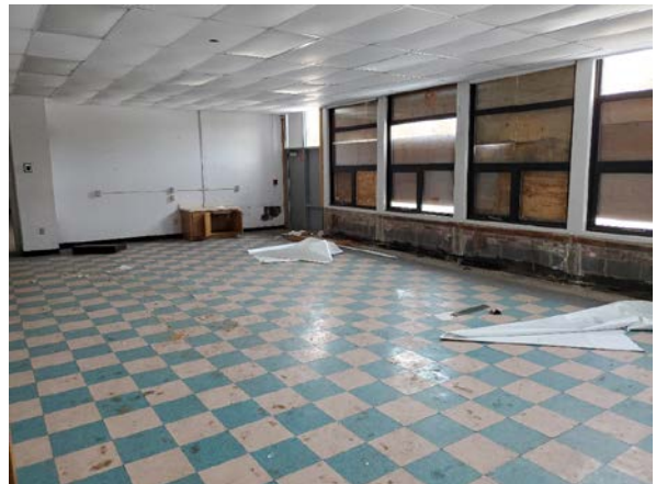
Photo 12: View of a 1 st floor classroom (typical) within the classroom wing addition to the building on the TP.
