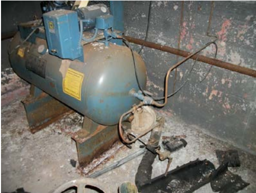
Photo 7: View of ACF Compressor in boiler room basement in original building on the TP.
