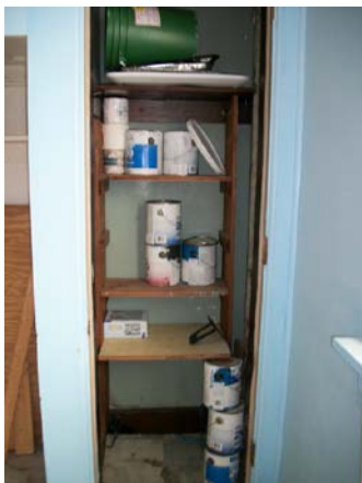
Photo 5: View of closet with 1-gallon cans of paint in 1 st floor classroom in original section of building on the TP.
