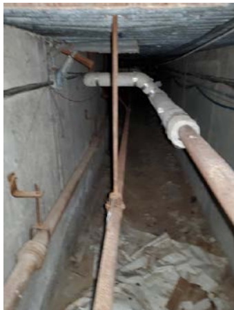
Photo 11: View of crawl space from 1 st floor surface entryway within the original building on the TP.
