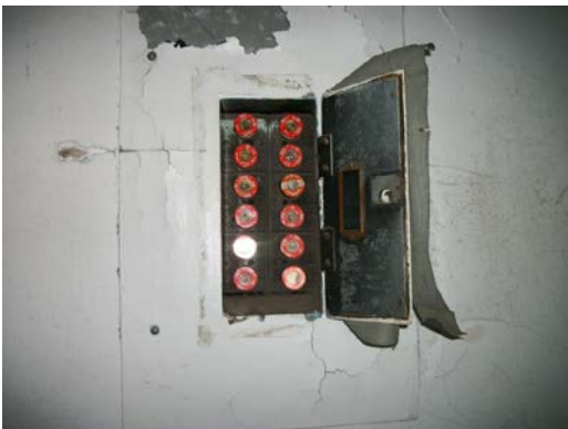
Photo 3: View of circuit breaker (typical) in original section of building on the TP.
