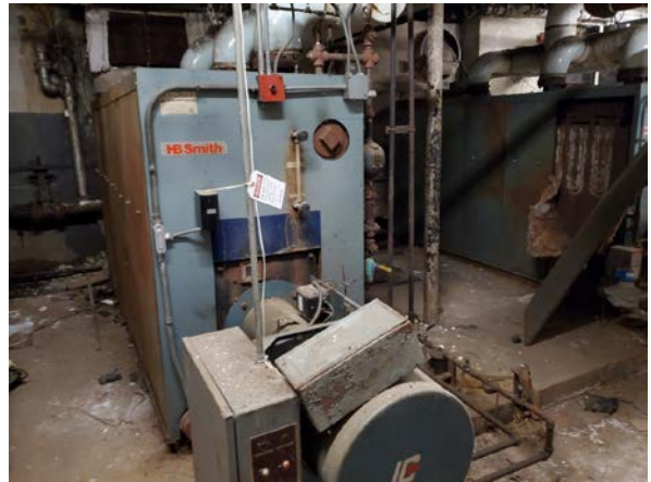
Photo 10: View of HB Smith Boiler (Series 28-1; N87 1019) in the boiler room of the original building on the TP.
