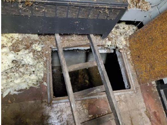
Photo 13: View of crawl space from 1 st floor entryway within the classroom wing addition to the building on the TP.
