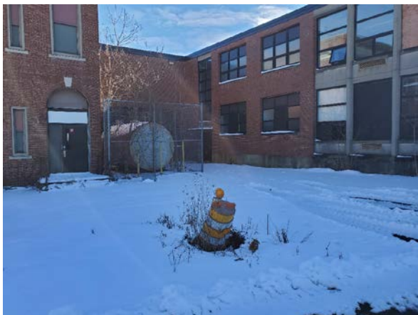
Photo 17: View southeast of subsidence near a catch basin (orange barrel) and with 6,000-gallon AST in distance at original / addition to building on TP.
