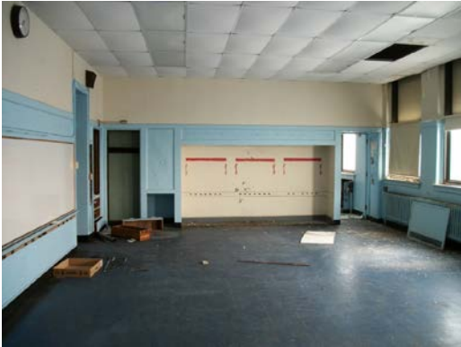
Photo 1: View of 2 nd floor classroom (typical) in original section of building on the target property (TP).
