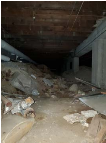
Photo 9: View north from the boiler room beneath the crawl space of the original building on the TP.
