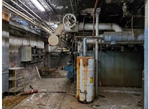
Photo 8: View of hot water tank in boiler room basement in original building on TP.
