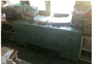
Heating and Ventilating units
