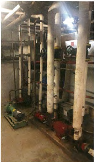
Hot Water System
